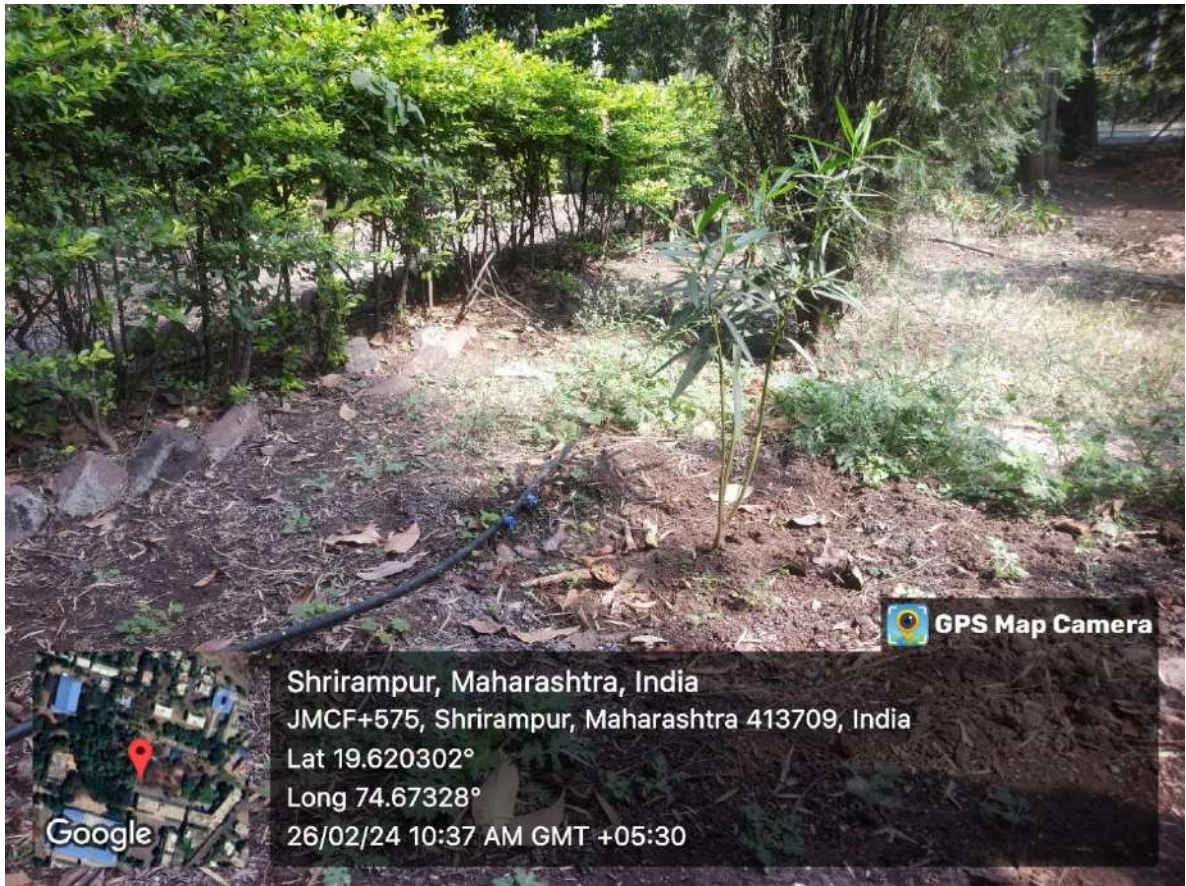
Water distribution to garden through Sprinklers and Drips
