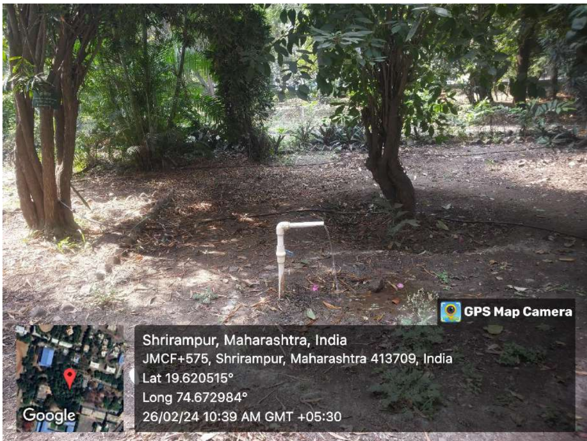
Underground Pipeline system for watering the plants in Botanical Garden
